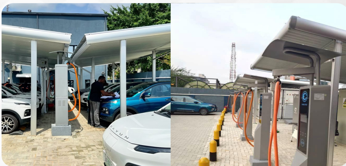
Figure 4: Folti EV Charging Infrastructure.
